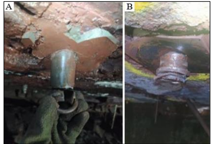
Fig. 5. (A) Total rupture of split set steel. (B) Ring deformation and beginning of weld breakage.
