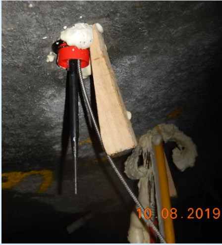
Fig 2: An installed 1 for radio
