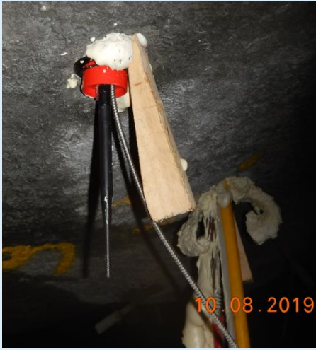
Fig 3: An installed 1 for 1 radio
