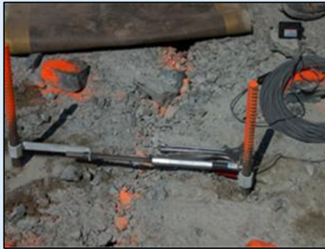
d-GMM used to monitor crack opening in the wall of the Dome Pit in Timmins.
